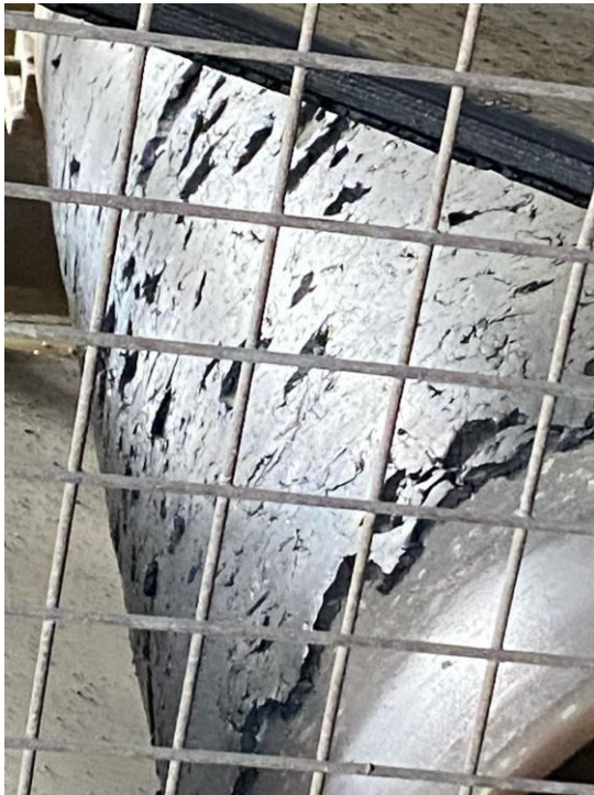
Before the repair
